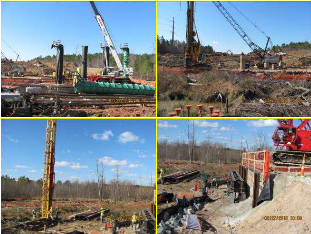
Picture 1: Pouring columns at Interior Bents 1 & 2 Picture 3: Driving temporary H-Piles for trestle bridge foundation
