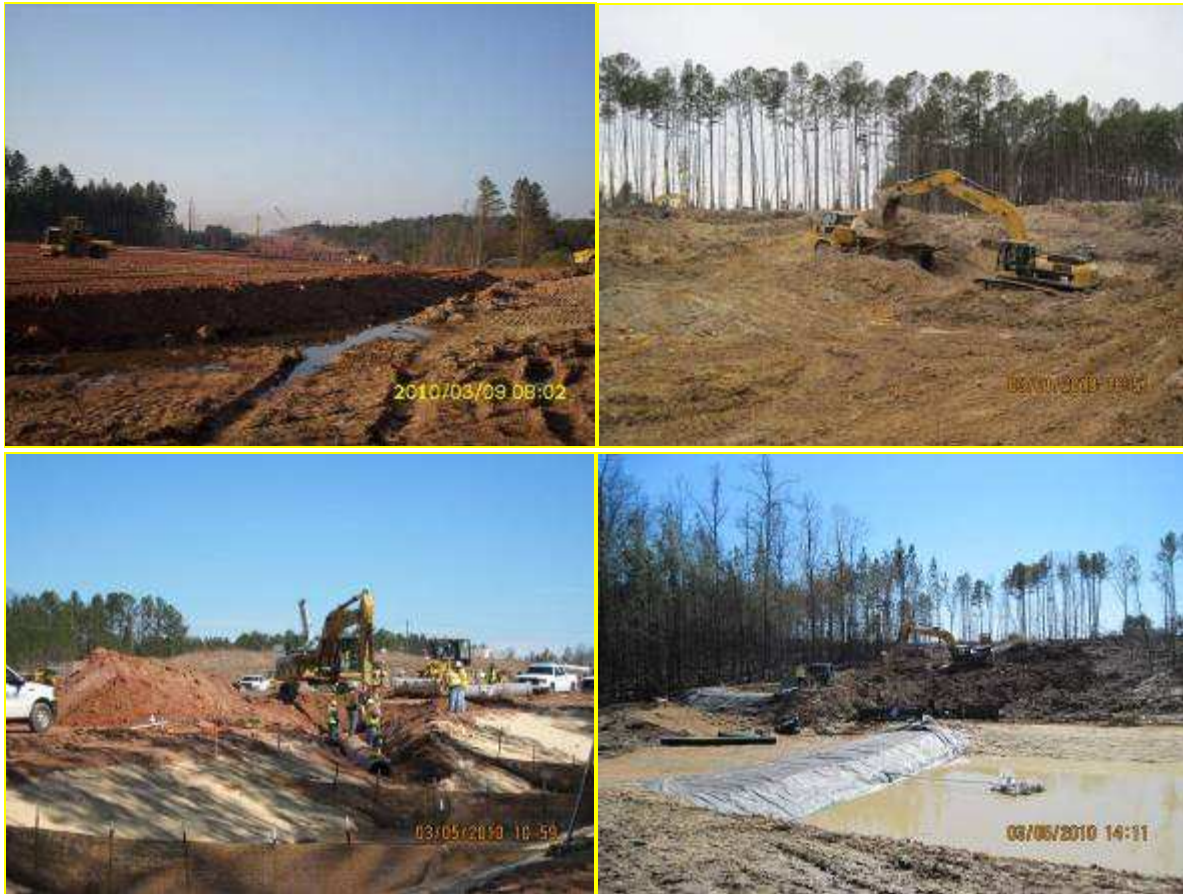
Picture 1: Excavation to embankment around Nancy Branch Picture 3: 24" CMP South of NC 55
