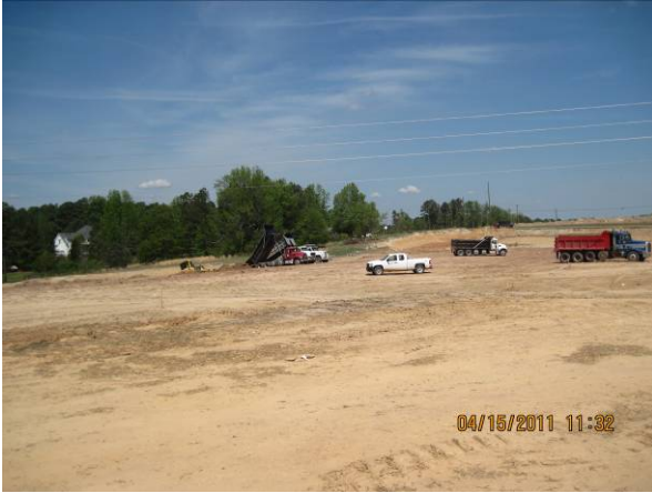
Embankment North of US64
