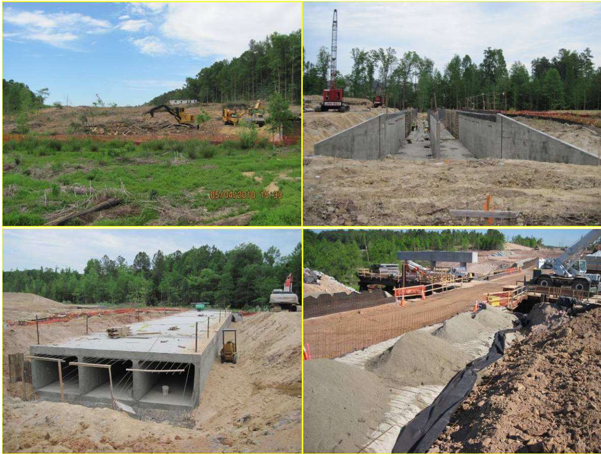
Picture 1: Clearing & Grubbing between White Oaks & Jack Branch Picture 3: Box Culvert No. 14
