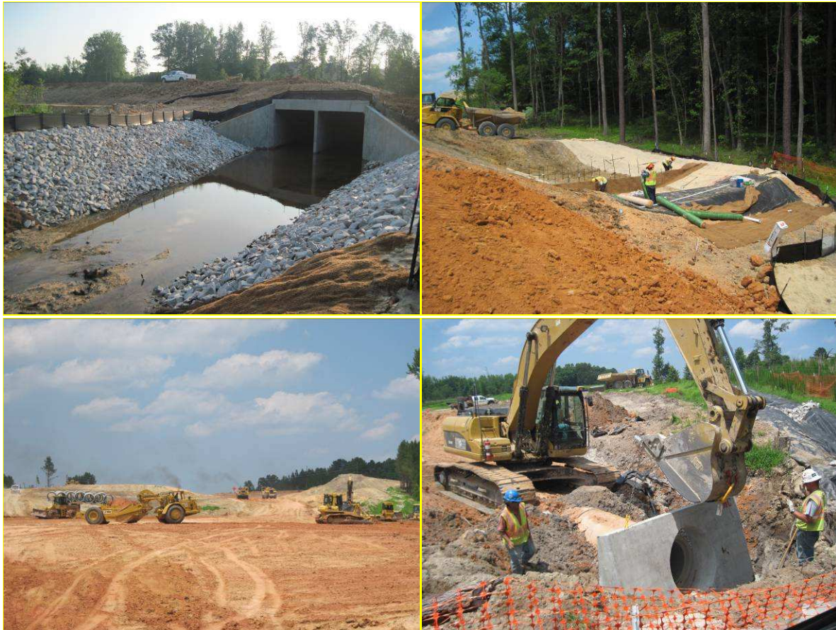
Picture 1: Channel Improvement at Box 13 Outlet Picture 3: Mass Haul South of Roberts Rd
