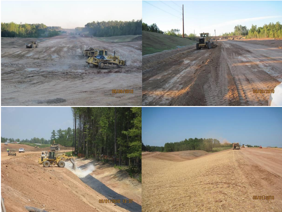
Picture 1: Eutaw Cut and Fill north of Green Level West Rd Picture 3: Installing Permanent Rip rap ditch C13
